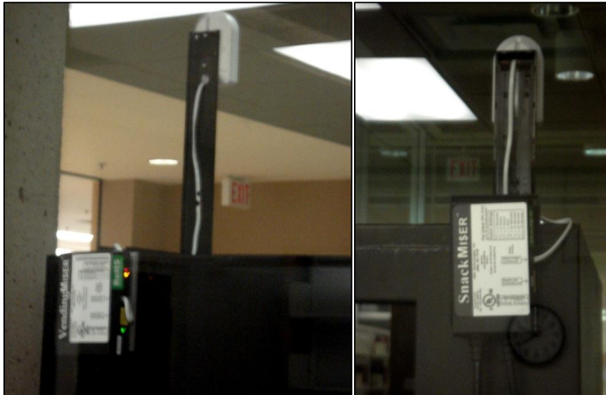
Figure 4: Vending Miser & Snack Miser Installed in Koerner Library (back view)
