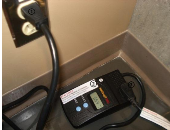
Figure 6: Power Connection with Watts Up? Meter Setup & Anti-Tampering Signs
